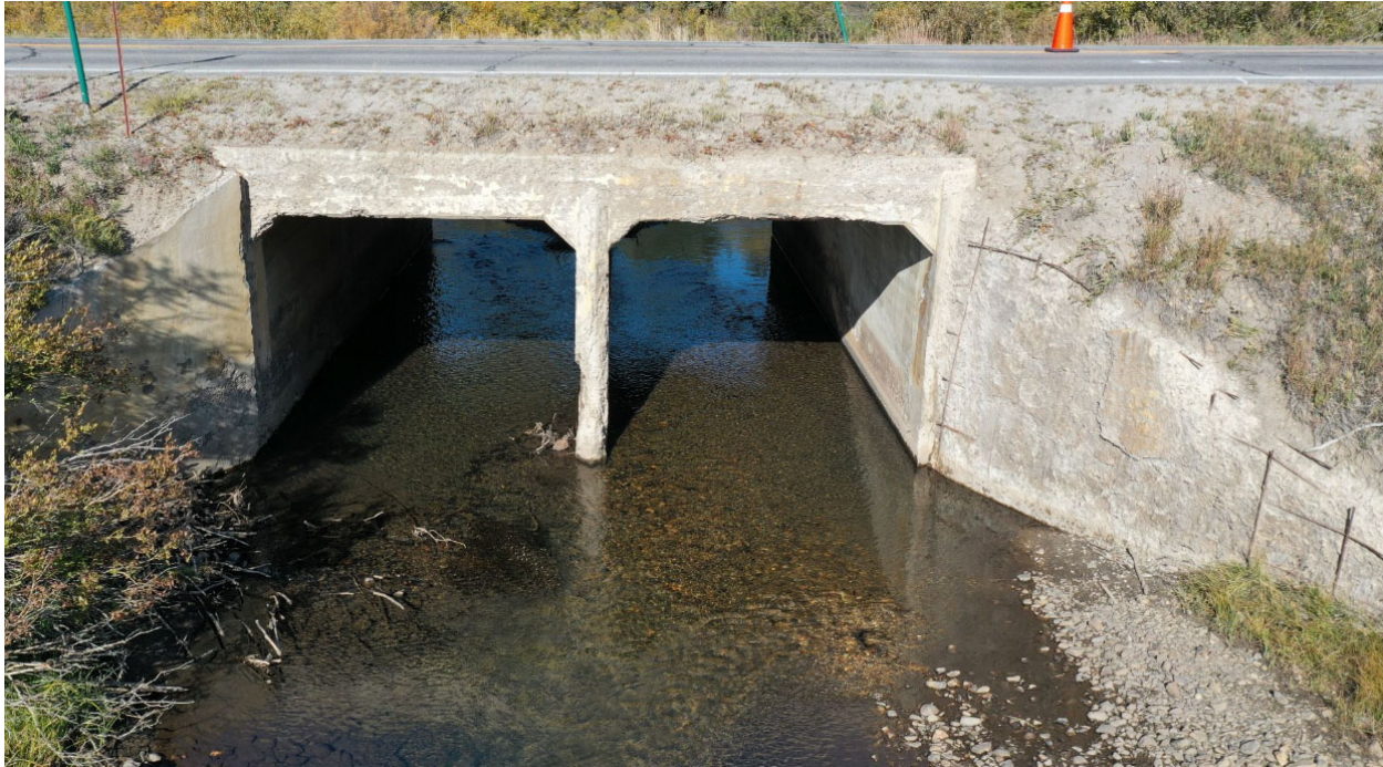
Picture 3 – Wingwall Exposed Reinforcement
