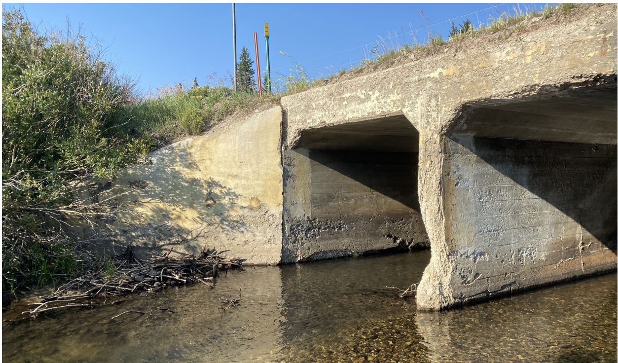
Picture 2 – Center Wall Loss of Section
